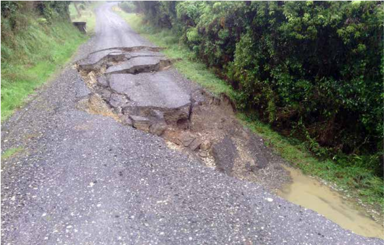
STORM DAMAGE TO PAEKAKA ROAD, PIOPIO - 5 APRIL 2017.
