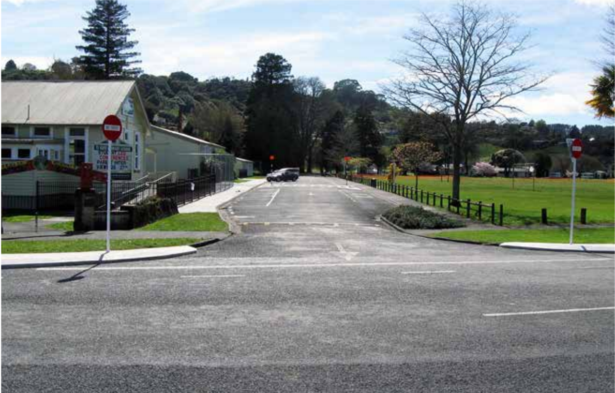
WORK COMPLETED IN THE VICINITY OF TE KUITI PRIMARY SCHOOL, TO IMPROVE THE POSITION OF THE CAR PARKS AND FOR THE PURPOSE OF ROAD SAFETY.
