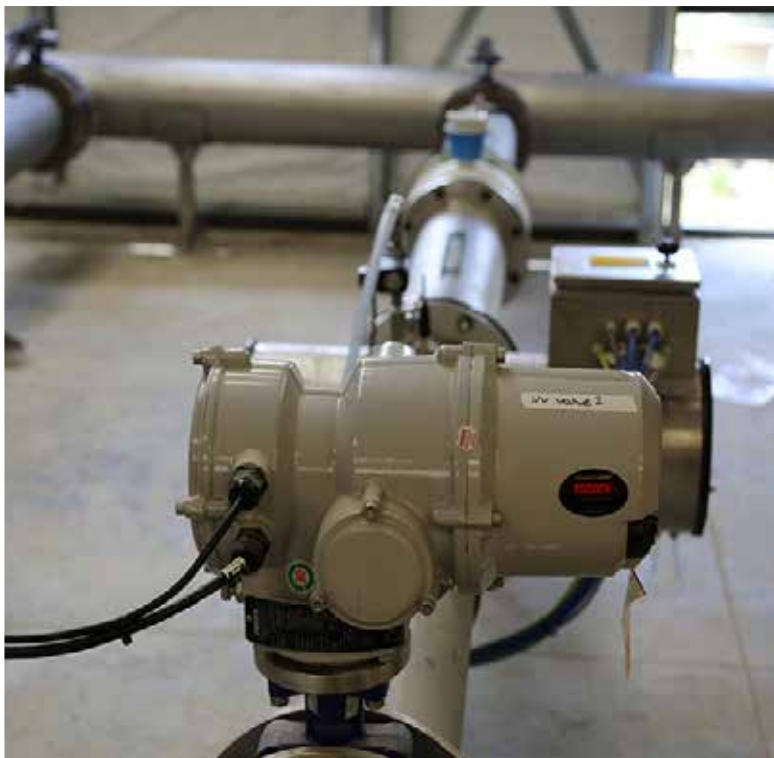
ULTRAVIOLET FILTRATION SYSTEM INSTALLED AS PART OF THE TE KUITI WATER TREATMENT PLANT UPGRADE
