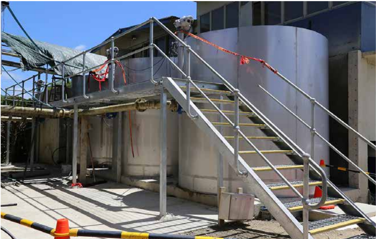
THE NEW STEEL WATER FILTERS WERE INSTALLED AS PART OF THE TE KUITI WATER TREATMENT PLANT UPGRADE
